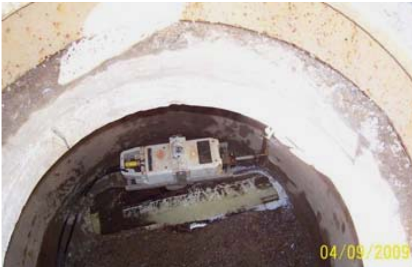
DDS Flo-Dar Sensor monitoring flow in 8" Sewer Line
