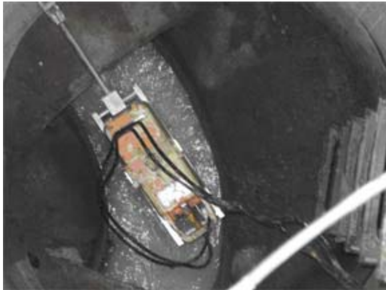
24" Sewer Line (Dublin Rd) Monitored by DDS Flo-Dar
