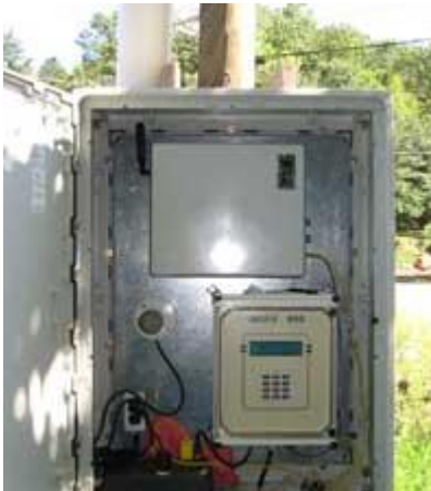
DDS Sigma Model 980 located at the entrance to the treatment plant on Hays Hollow.
