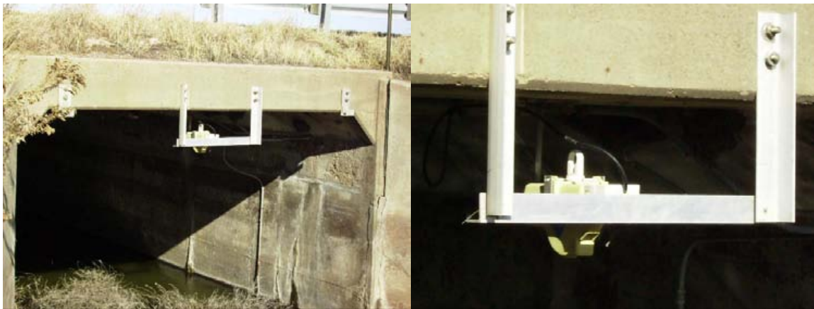
Flo-Dar Sensor installed in a box culvert application at Cheyenne Bottoms Wildlife Area
